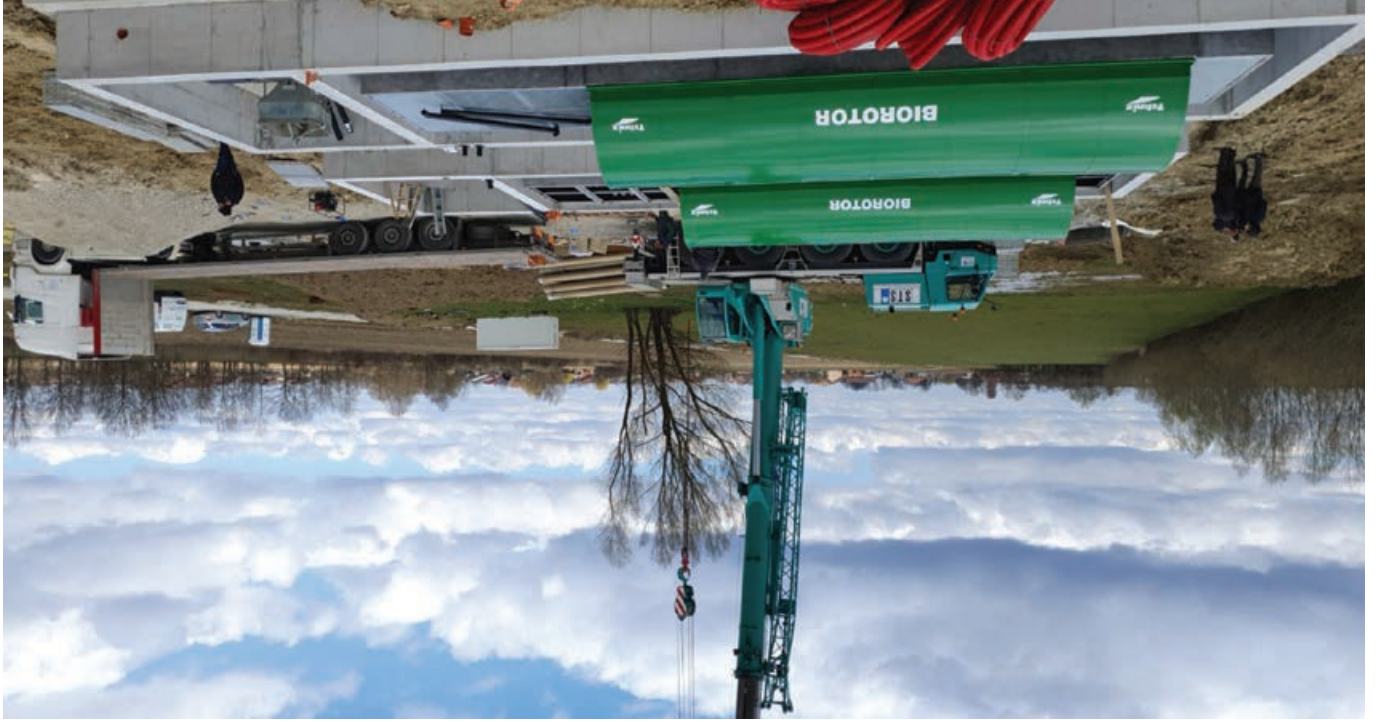
INSTALLATION OF THE TEHNIX BRT - 2000 ES BIOROTOR WITHIN THE SCOPE OF THE WASTE WATER DRAINAGE AND TREATMENT PROJECT FOR THE BRESTAČA AND NOVA SUBOCKA SETTLEMENTS FOR THE TOWN OF NOVSKA
